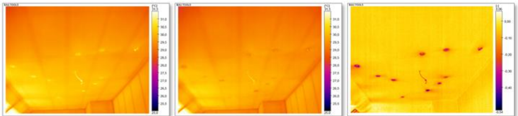
Leaks in recessed ceiling spotlights (downlights)
